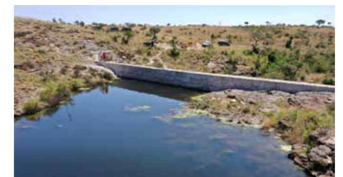
Nanja North Weir A: The completion of Weir A will add 7.5 million litres of water to Mpala.
